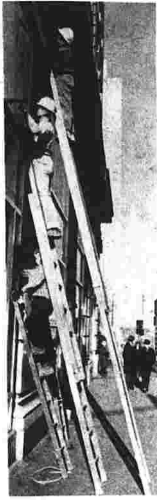
THREE MAY BE a crowd in some circles, but for building maintenance men in Wilmington, Del., it gets a job done faster, and saves a lot of ladder raising and lowering.
